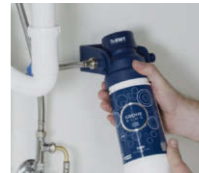
Attach filter holder to the cabinet and screw filter into filter head. Then connect the filter to the cold water supply.
